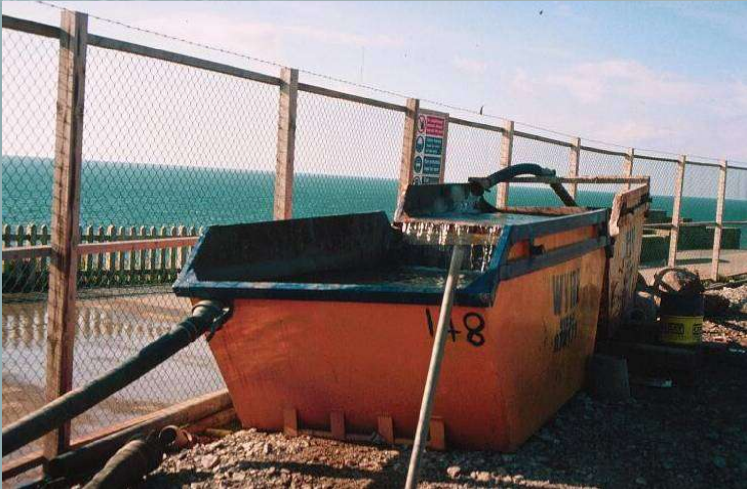
Simple skip arrangement used as settlement tank
